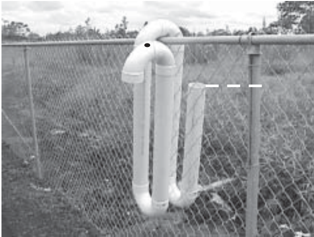
An overflow device to keep the water level as indicated. Pipe on the near side of the fence hangs outside the tank. A hole atop the elbow in the foreground is needed for proper function, but if a T-joint is used, the hole is not needed.
