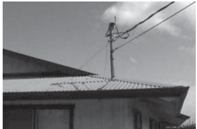
Rodents can access your roof by climbing utility poles and running along electrical and phone cables. Putting the wires underground is an expensive but good solution to the problem. Attaching the wires to the side of the house may be an option if the house is tall enough to keep the wires out of reach. Contact your utility companies for advice.
